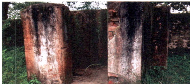
Deplorable and non-functional toilet at Madanpur PHC
